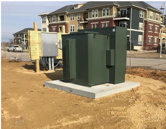
Above: The temporary power transformer has been installed for the job office trailers and the site needs. With a project this size, there will be multiple transformers to meet the power demand for construction.
