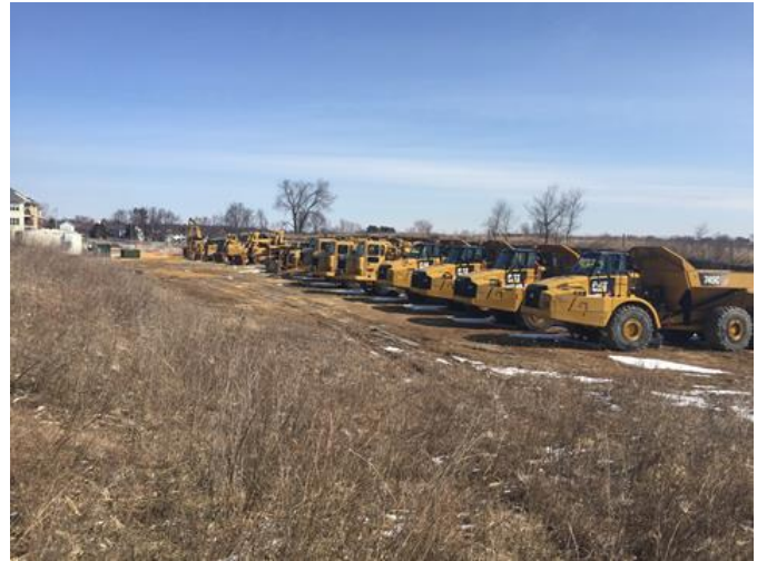
Start your engines! Earthwork subcontractor Mashuda has a long line of equipment ready to start grading for the new Verona Area High School.
