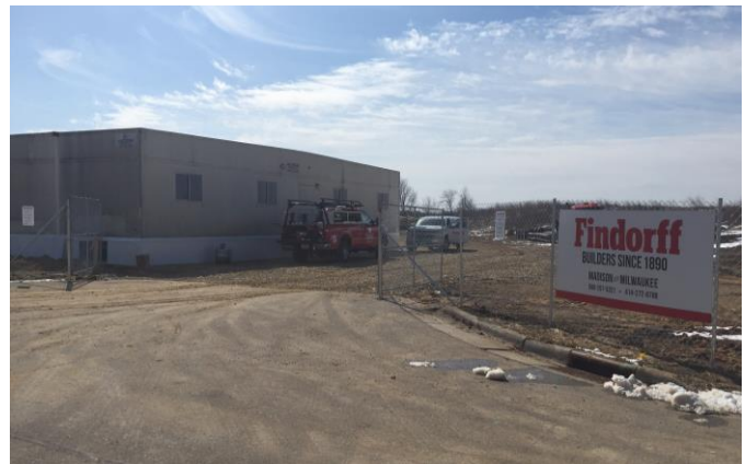
The temporary construction fence was installed last week and the job office trailers have been placed.
