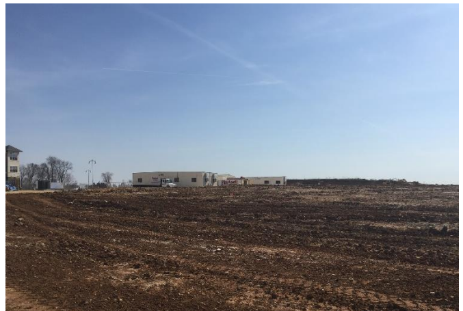
The large pile of dirt located behind the tent and podium during the ground breaking ceremony is gone! The site looks different almost everyday as Earthwork subcontractor Mashuda moves about 16,000 cubic yards of dirt a day!
