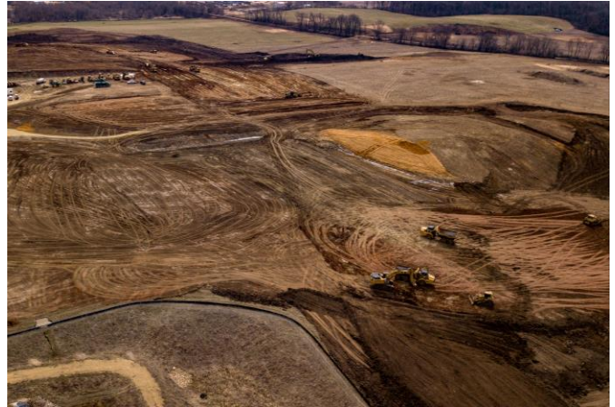
The photo above shows an aerial view of the site from last week Thursday. Where the earth has been disturbed the future school, parking lots, and football stadium will be located.
