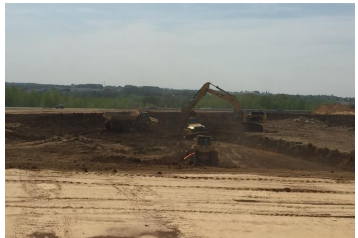
That is a deep hole! The Earthmoving contractor Mashuda has been busy with the over excavation in the future Pool and PAC area.
